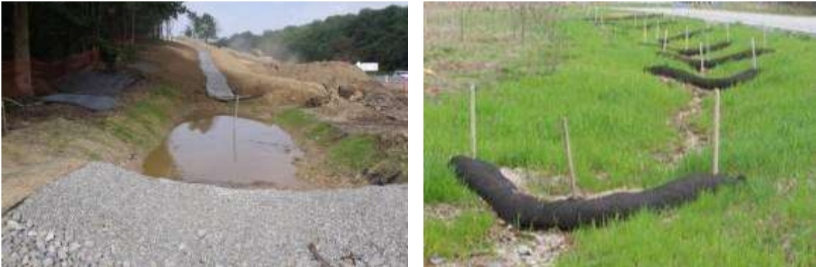
Figure 49: Erosion and sedimentation control - sedimentation basins
