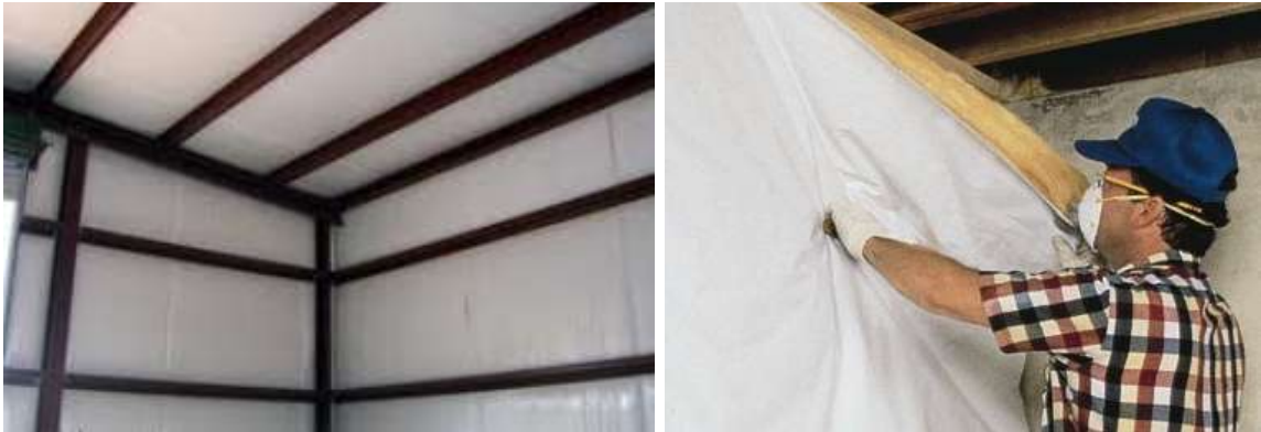
Figure 62: Faced MBI fiberglass wall
